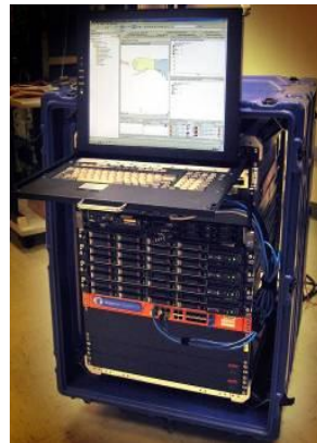
Targeted attack monitoring system
