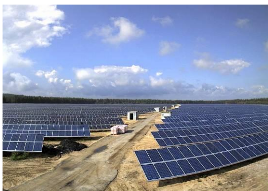
Solar power generating facility in Germany
