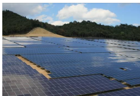
-Solar power generation equipment supplied to Taihan Techren Co., Ltd.
