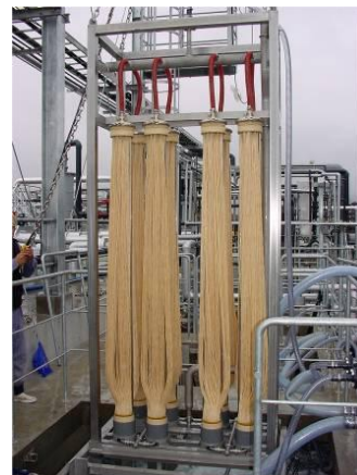
-Waste water treatment and recycling membranes
